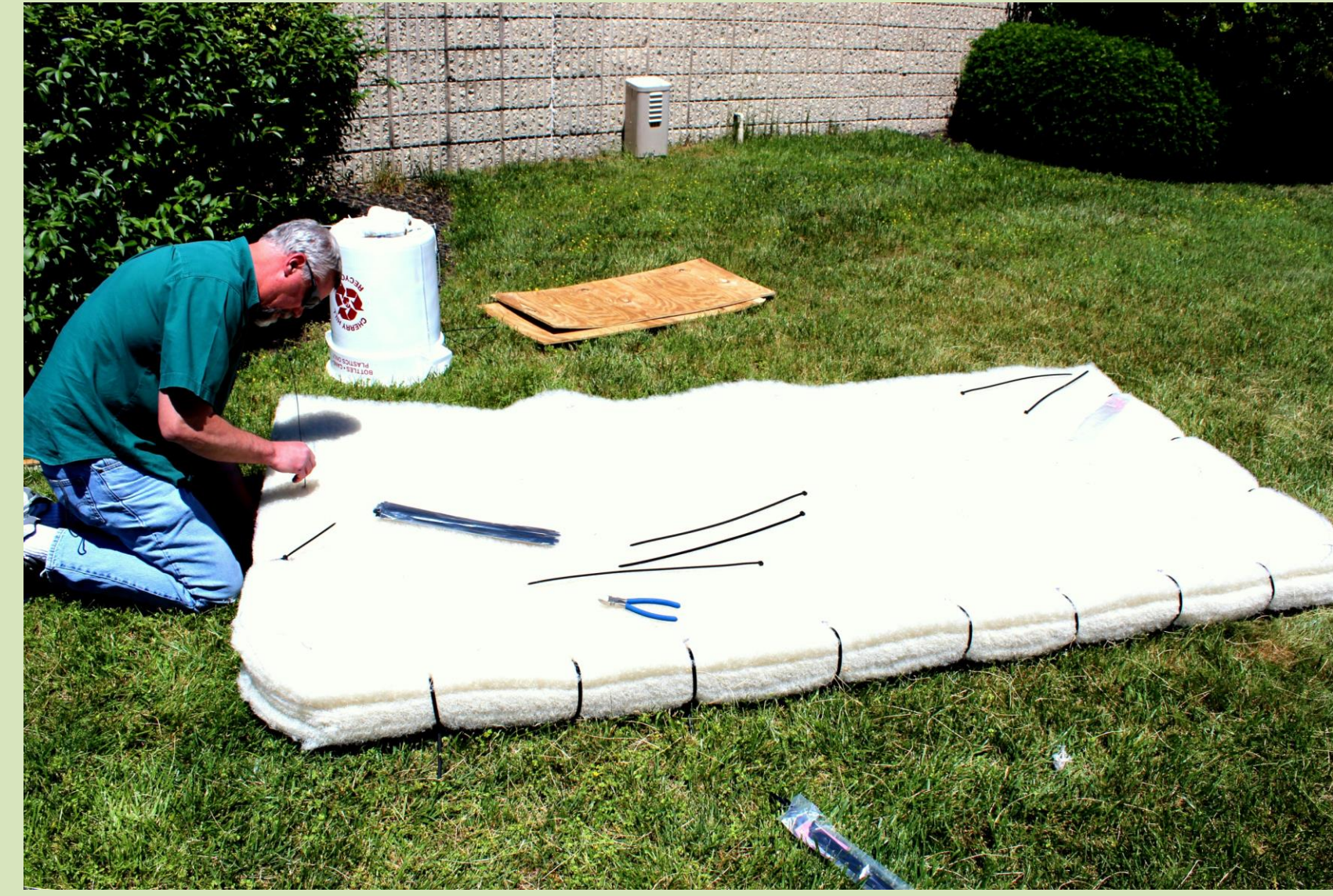
Forming the base by zip tying 3 layers of Poly-Flo filter material together.
